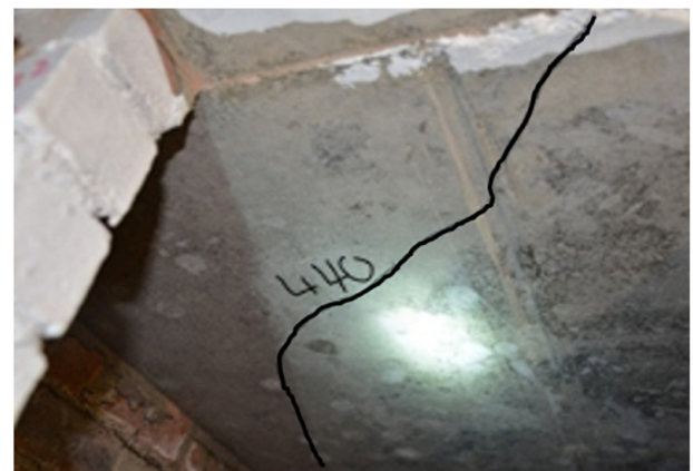
(b) Cracks extended to the slab
