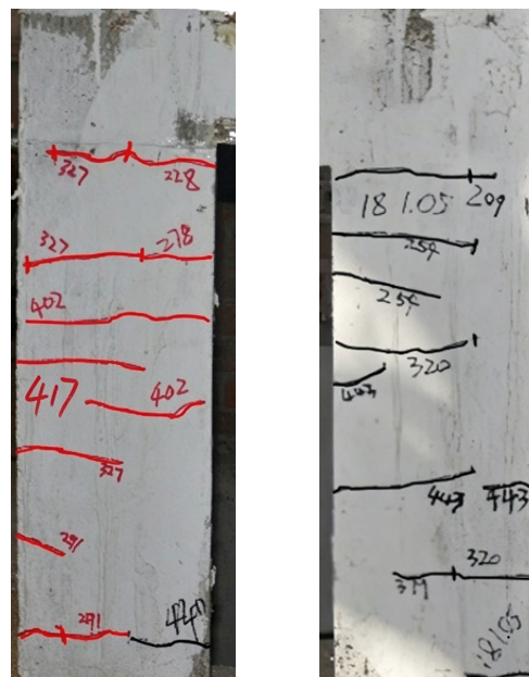
(a) Cracks in wall Q1 (b) Cracks in wall Q5
