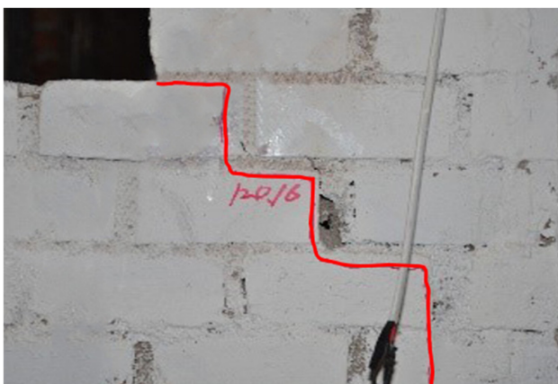
(a) Cracking on the longitudinal wall
