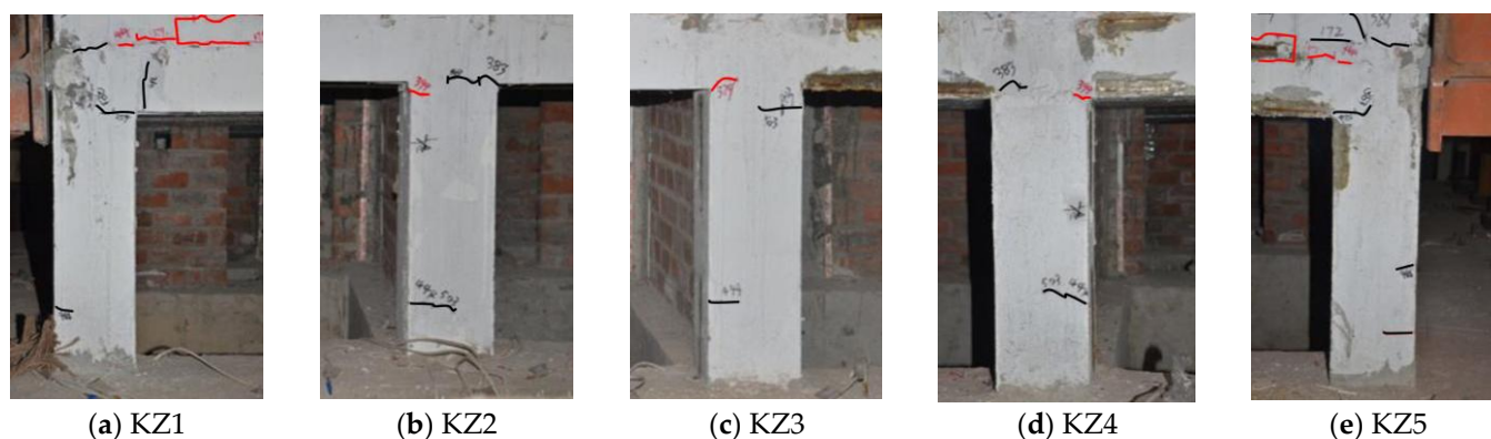
Figure 13. Crack pattern of the frame columns at the ground-level floor along A-grid line.
