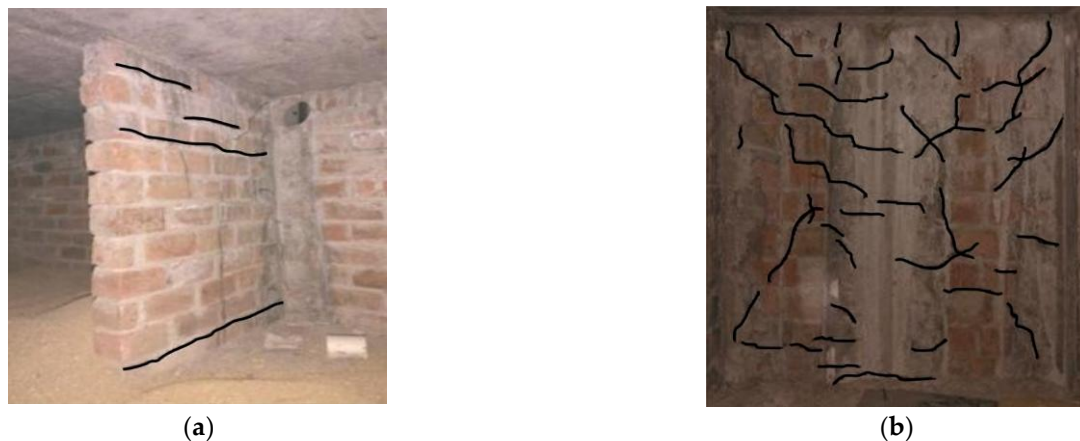
Figure 18. Crack pattern of the longitudinal walls and constructional columns along B-grid line. (a) Wall limb and constructional column on the ground-level floor of 9-grid line. (b) Wall limb and constructional column on the third floor of 5-grid line.
