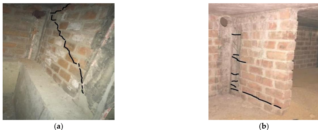
Figure 19. Crack pattern of the longitudinal walls and constructional columns along C-grid line. (a) Wall limb and constructional column on the ground-level floor of 1-grid line. (b) Wall limb and constructional column on the second floor of 1-grid line.
