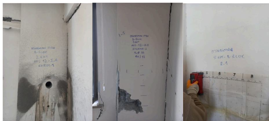
Figure 11. Experimental study in the investigated building.
