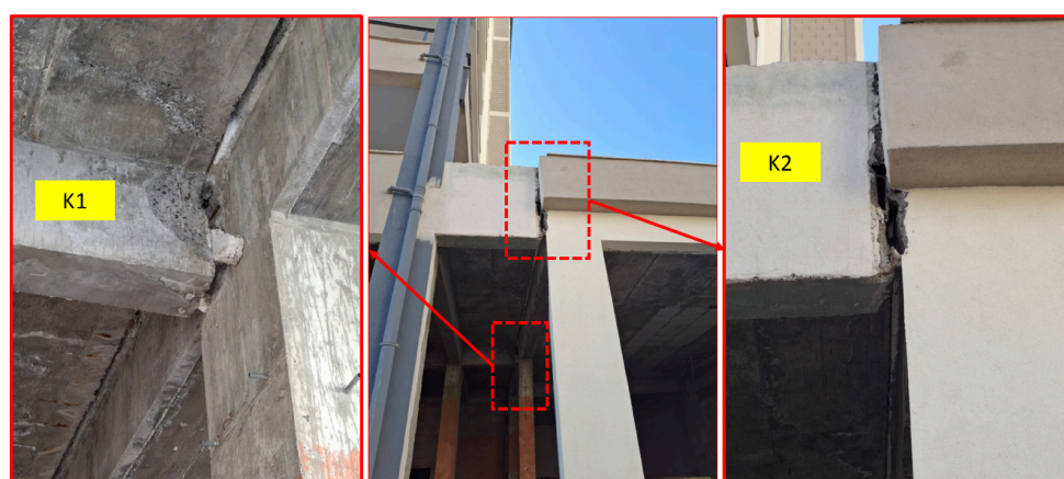
Figure 10. Observed damage due to the pounding effect.
