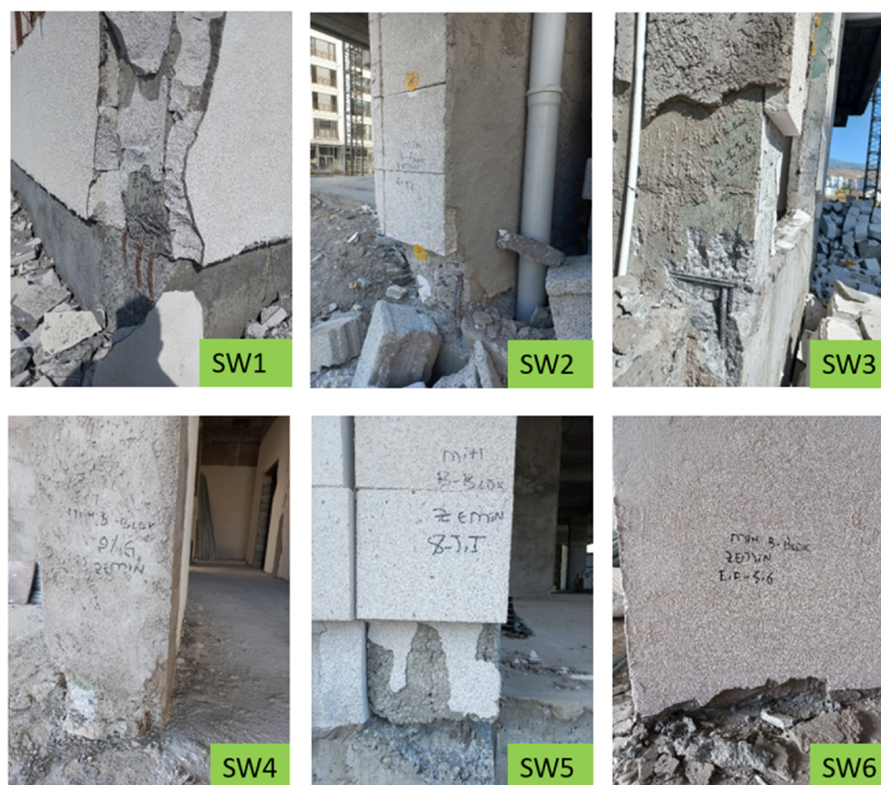
Figure 9. Structural damage to the shear walls on the ground floor.
