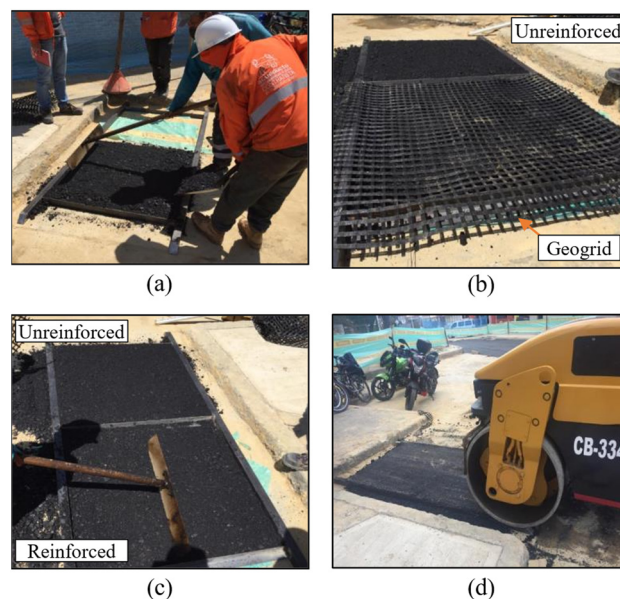
Figure 3. Test sample fabrication process: (a) area demarcation, (b) location of the geogrid, (c) the second asphalt layer, and finally (d) the compaction process.
