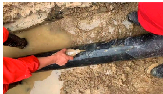
Figure 1. Photo of the pipeline failure site.
