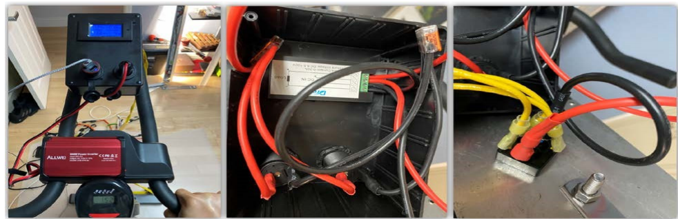
Figure 10. The electrical components on the prototype.
