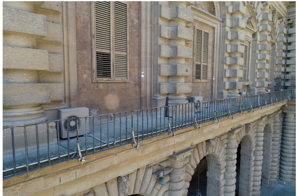
Figure 19. Air conditioning systems on the terrace of the second floor. Such elements can be wrongly classified.
