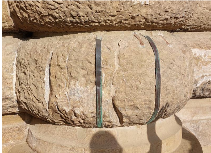
Figure 4. An example of a broken ashlar fixed with several types of metal ties over time.
