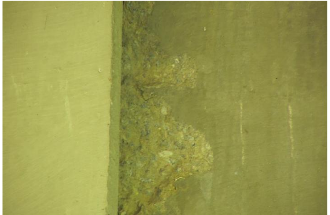
Figure 4. Minor spalling observed DJI M210 RTK drone [68].
