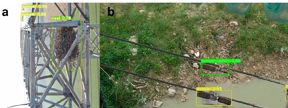
Figure 9. (a) Bird nest identification, (b) damper defect identification.
