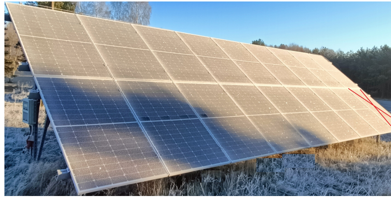
Figure 3. Stationary PV installation.
