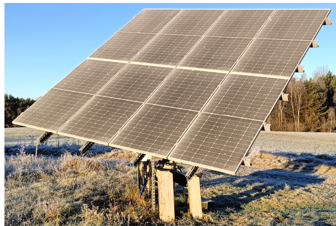
Figure 4. Tracking PV installation.
