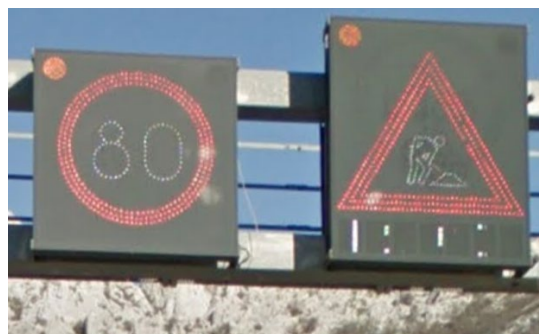
Figure 2. Variable message signs (VMS) on a Croatian A1 motorway designed as electronic LED panels.
