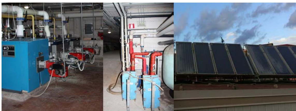
Figure 3. Main components of the swimming pool existing installation: natural gas boilers ( left ), swimming pool heat exchangers ( centre ), thermal solar collectors ( right ).
