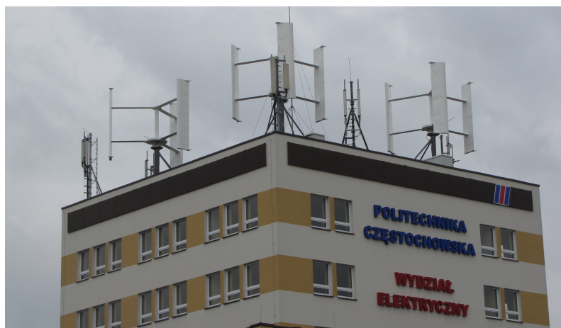
Figure 4. The FEE 30 kWp wind power plant.
