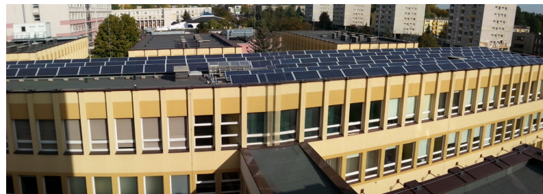
Figure 3. The FEE 45 kWp photovoltaic power plant.
