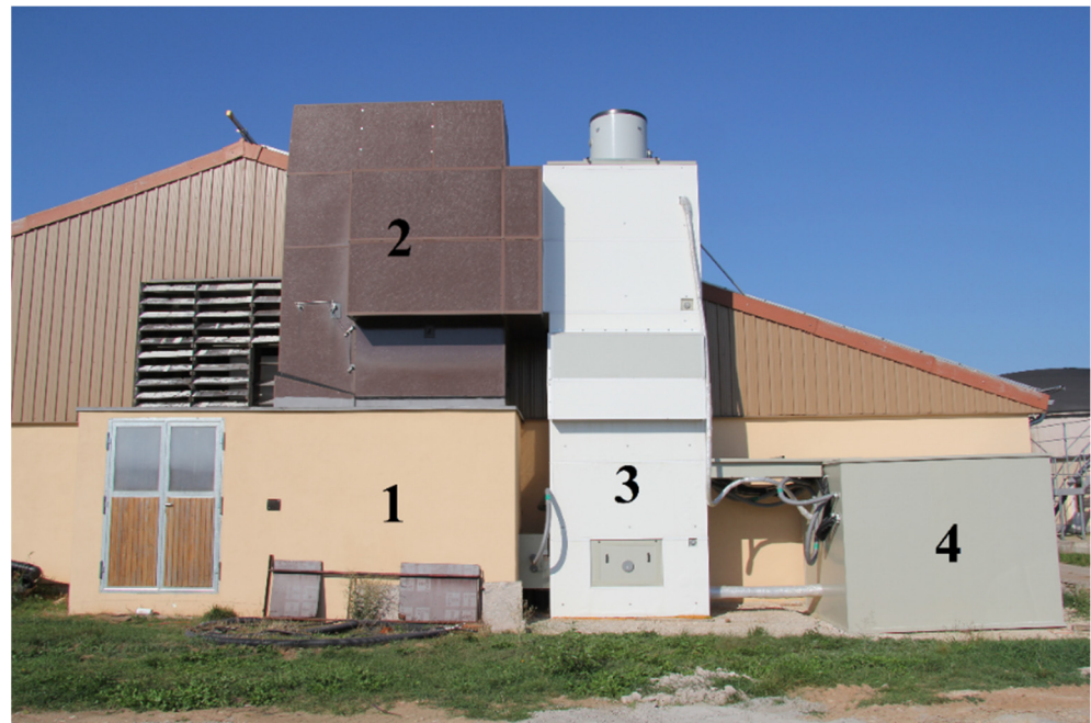
Figure 1. External view of the exchange scrubber pilot plant. Part of the exhaust air is drawn from the vacuum chamber (1) below the conventional heat exchanger (2) into the pilot plant (3). To the right of the test pilot plant is the equipment container (4), which housed the scrubbing water basin, the exhaust air treatment technology and its controls, as well as all measuring technology.
