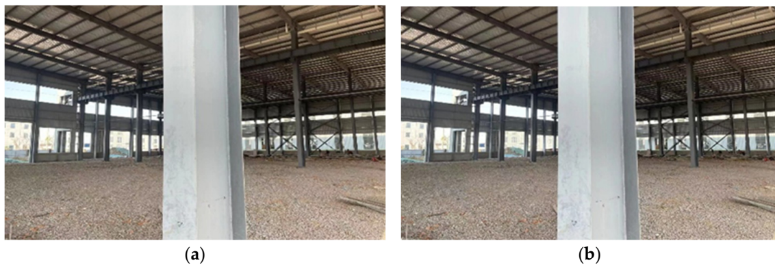
Figure 5. Original binocular images of steel structure column: (a) is left-eye image; (b) is right-eye image.
