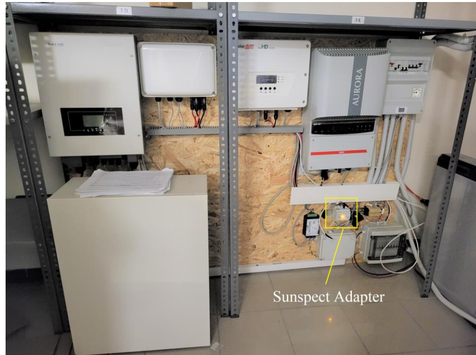
Figure 13. The 4 kW-4 kWh SolarEdge battery storage.
