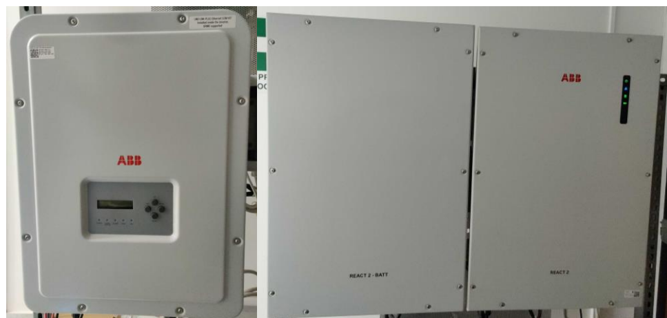
Figure 11. The 3 kW–12 kWh battery energy storage system, model React2, produced by ABB.
