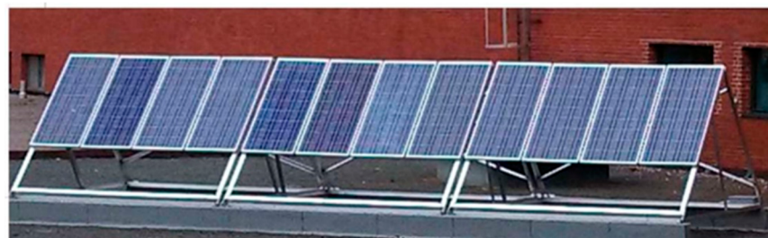
Figure 10. MUN ECE laboratory PV installation.
