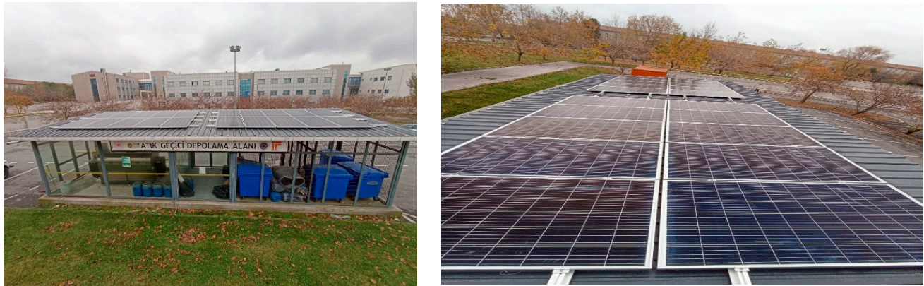
Figure 2. An off-grid solar energy system with 6.6 kWp installed capacity.
