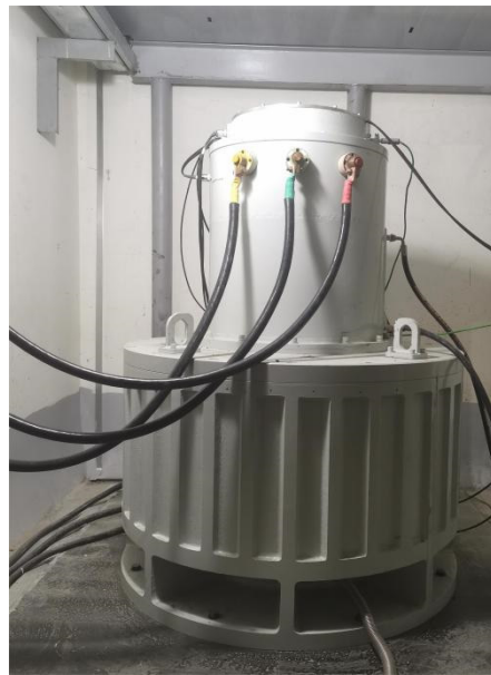
Figure 27. Flywheel energy storage unit placed underground.
