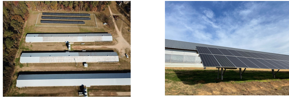
Figure 2. Two distributed photovoltaics systems of 180 kW ( left ) and 50 kW ( right ) installed on commercial poultry farms.
