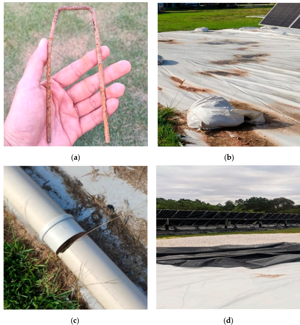
Figure 16. Problems identified in film fixation methods: (a) corrosion of metallic staples; (b) sand spreading from anchoring bags; (c) sand spreading from anchoring tubes; and (d) film detachment during a windy day due to insufficient fixation.
