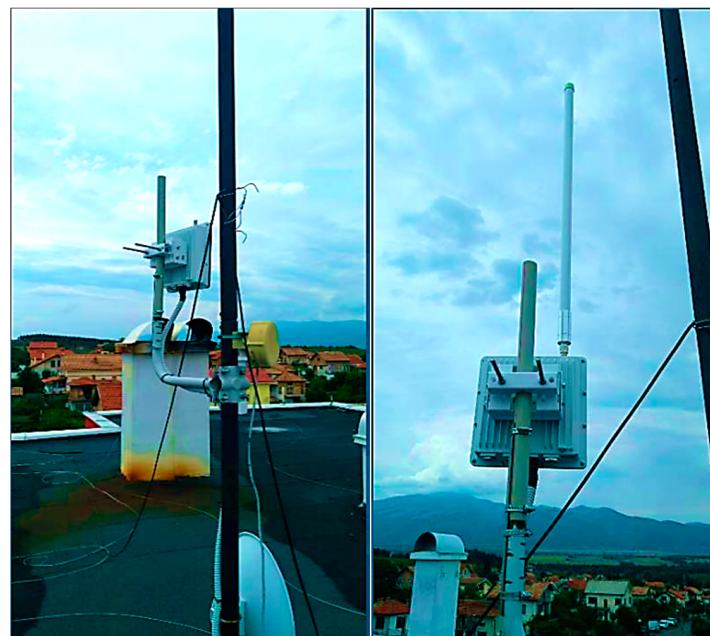
Figure 7. Installation site of the experimental LoRaWAN gateway.
