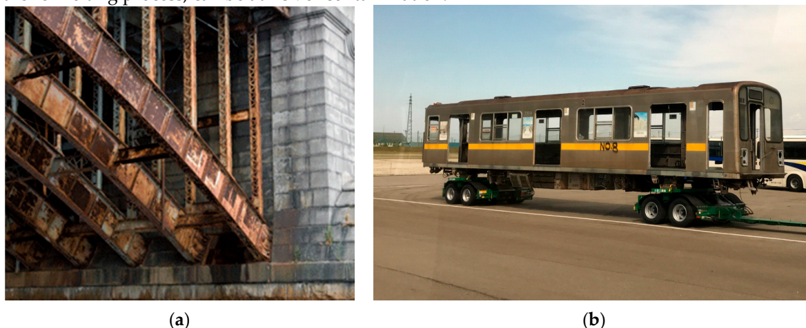
Figure 8. Corrosion of steel. (a) Extreme corrosion in a bridge. (b) Railway rolling stock being renovated.
