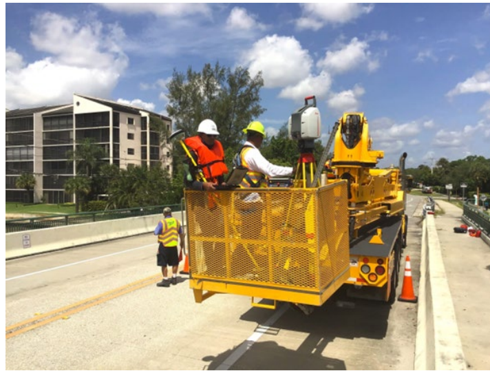
Figure 14. Leica scan station II set up in man basket of snooper truck used for underwater scanning of highway bridge—Little Lake Worth Bridge, Florida.
