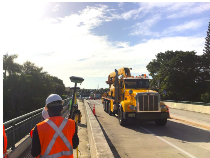
Figure 13. Snooper truck used for underwater scanning of highway bridge—Little Lake Worth Bridge, Florida.
