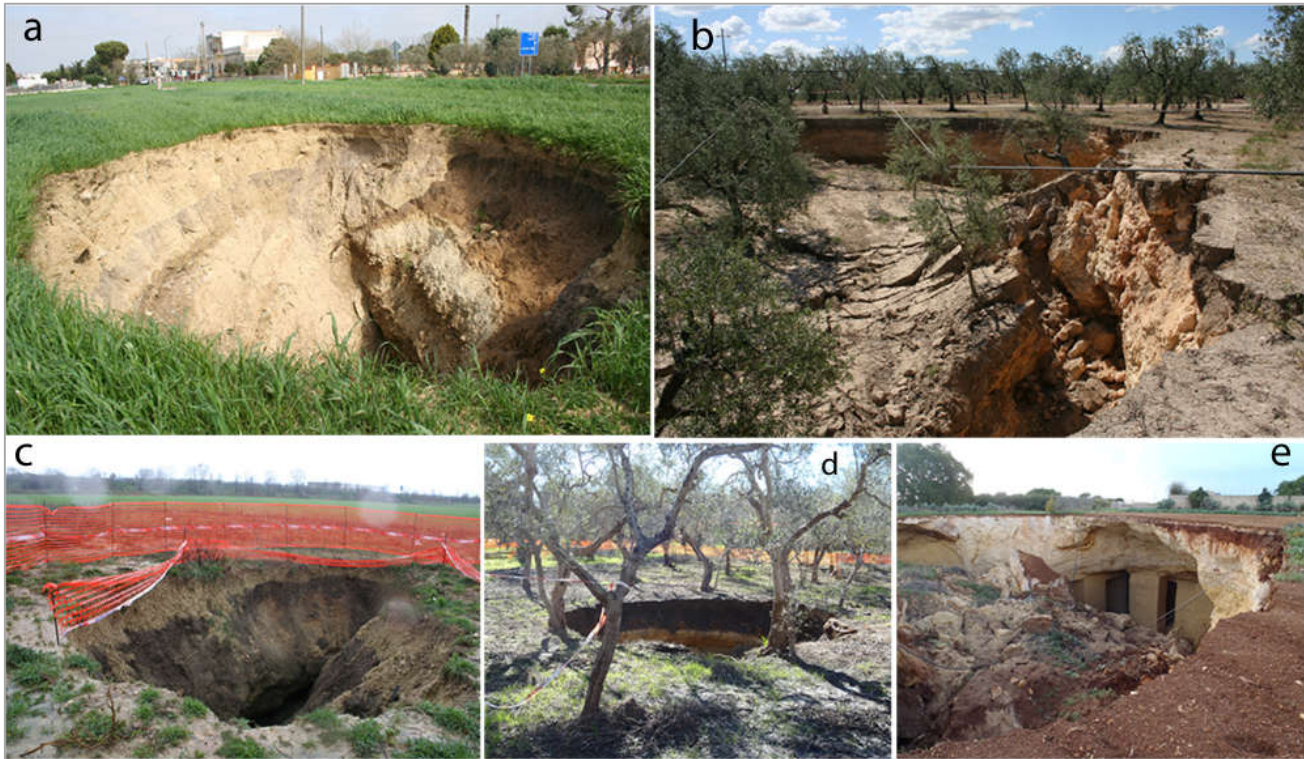
Figure 2. Sinkholes related to artificial cavities. All examples refer to underground calcarenite quarries, a rock material frequently used for building construction: (a) Cutrofiano, Apulia; (b) Barletta, Apulia; (c,d) Altamura, Apulia; (e) Marsala, Sicily.
