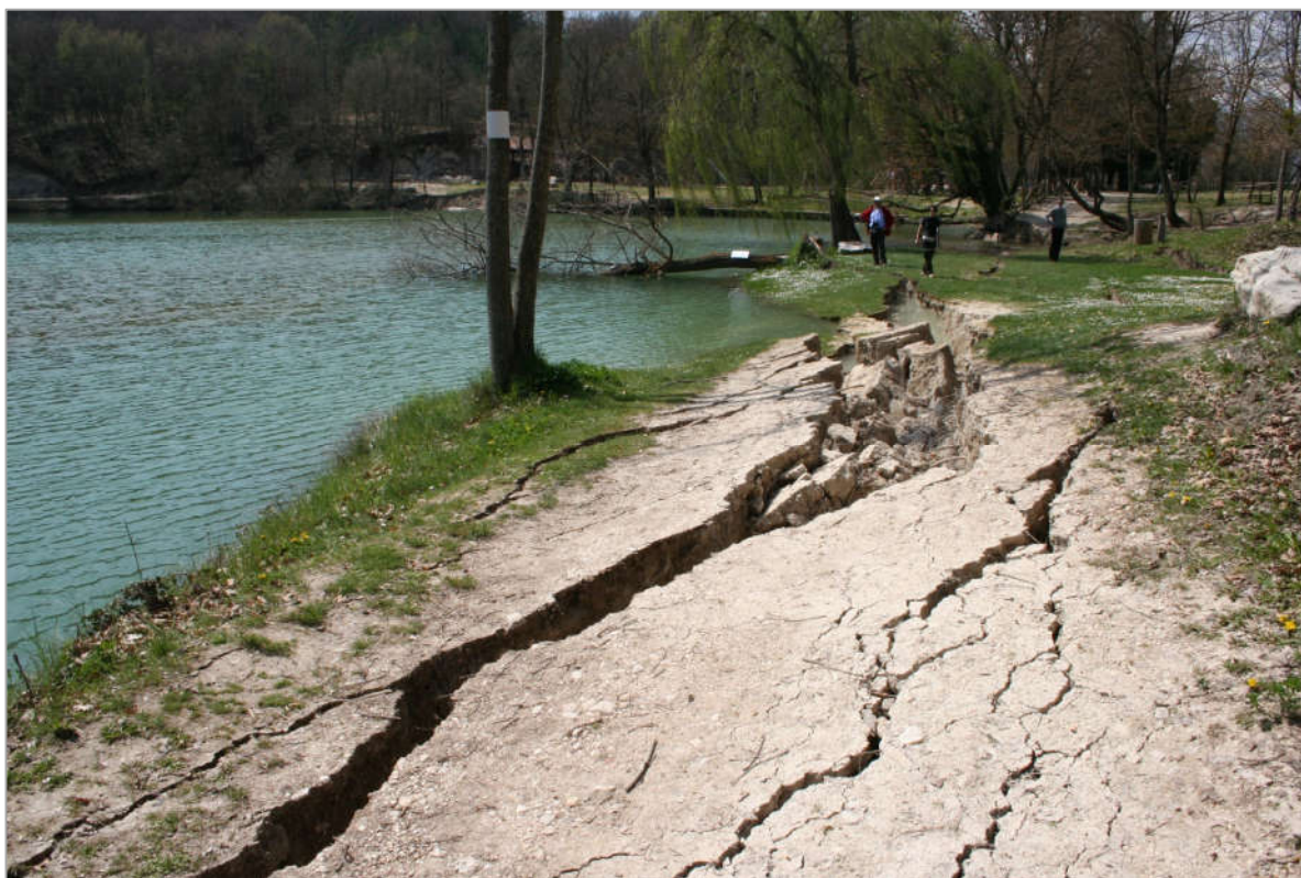
Figure 10. Open cracks and shore disruption at Sinizzo Lake (Abruzzo, Italy) after the L'Aquila earthquake on 6 April 2009 (Mw 6.3).
