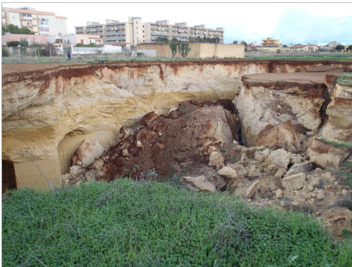
Figure 9. Sinkhole occurrence in urbanized areas can pose serious risks to society, threatening buildings and infrastructures.
