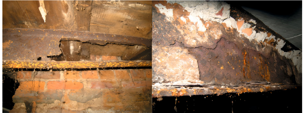
Figure 10. Deep corrosion damage of metal underground structures in the restored basement of an old residential building in Saint Petersburg (photo by I.V. Alekseev, 2016) [36].
