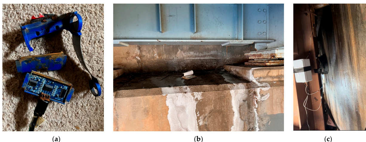
Figure 9. Glimpses of field environmental challenges: (a) Corroded sensor pins; (b) Flowing deicer through the joint; (c) Flowing water within the sensing system from the joint.
