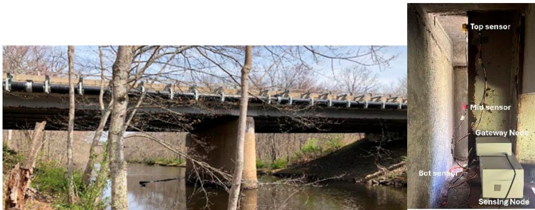
Figure 2. Photograph of Bridge 1 (CT NBI ID1531) (left) and field-installed monitoring system (right).
