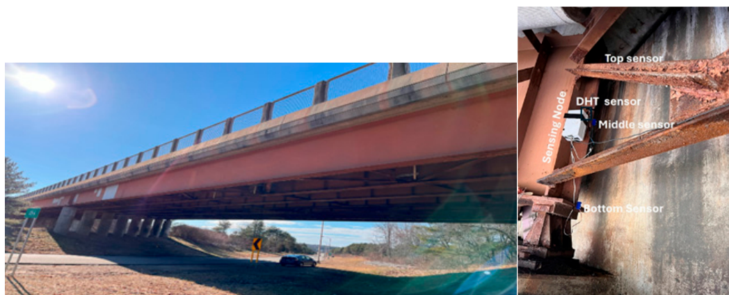
Figure 3. Bridge 2 (CT NBI ID2570) (left) and field-installed monitoring system (right).
