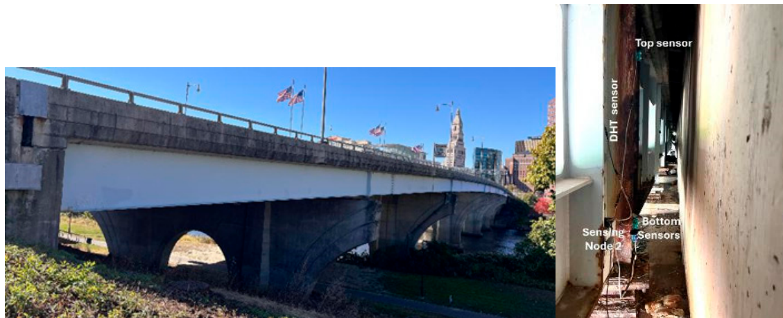
Figure 4. Bridge 3 (CT NBI ID0674A) (left) and field-installed monitoring system (right).
