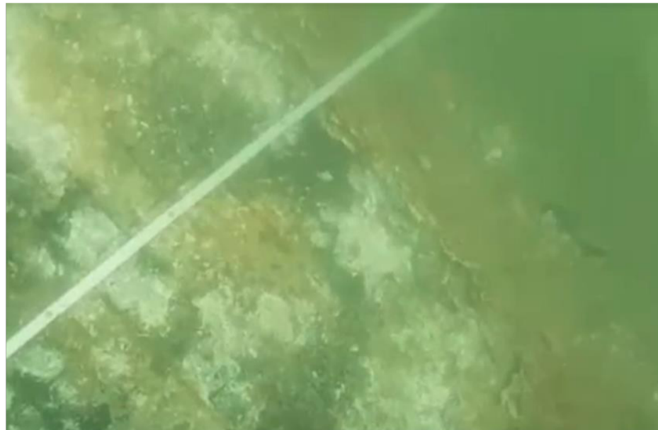
Figure 1. Typical example of the environment around a subsea pipeline (SP) and the condition of its outer surface (the SP is illuminated by the divers' powerful torches).
