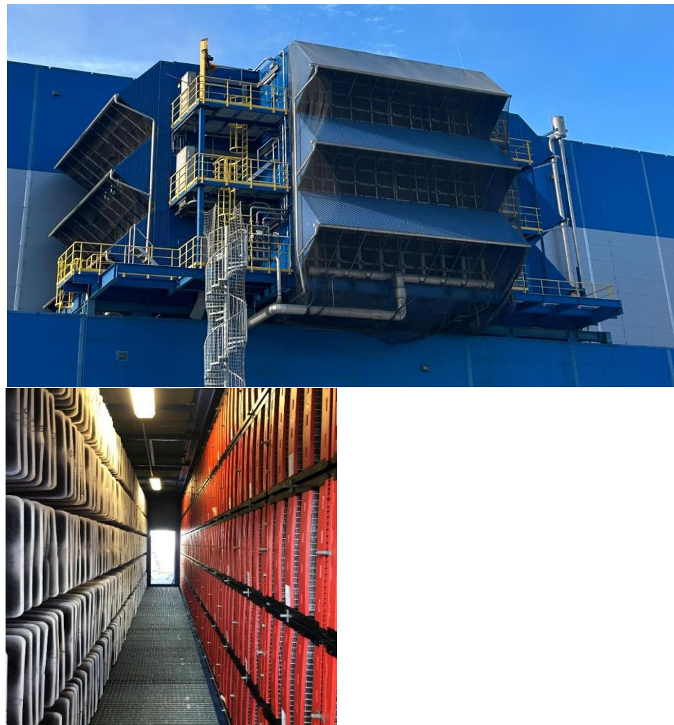
Figure 2. General views of the inlet air filtration system of the examined.
