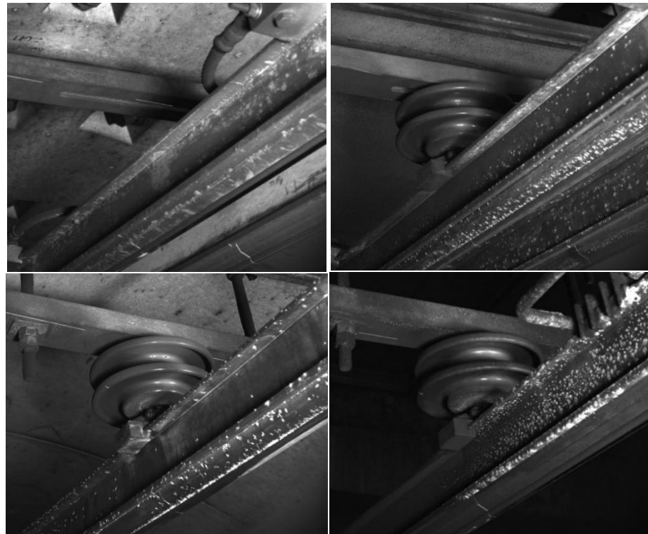
Figure 7. Chemical Corrosion of the Conductor Rail.
