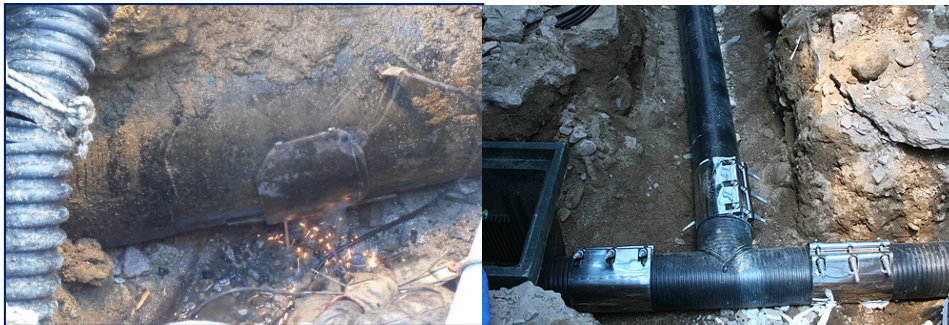
Figure 1. Failure of underground pipelines.
