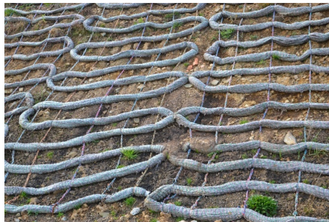
Figure 1. The segments of ropes arranged in a meander-like pattern that were installed on the slope.
