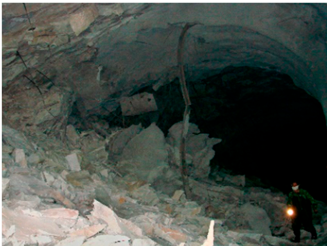
Figure 5. Supporting systems failure in underground tunnels following violent rockbursting and spalling due to instability of the reinforcement elements [46].
