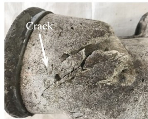
(b) Local failure of concrete
