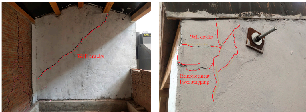
Figure 13. Failure mode of the east gable wall: (a) On the inside; (b) on the outside.
