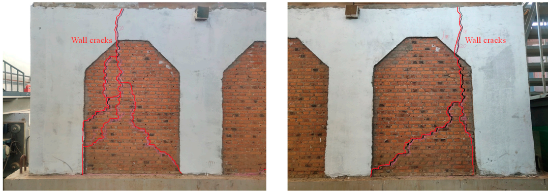
Figure 12. Failure mode of north elevation: (a) The east side; (b) the west side.
