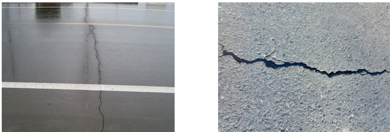
Figure 1. Top-down transverse cracks on the road surface and bottom-up reflective cracks on the base layer.
