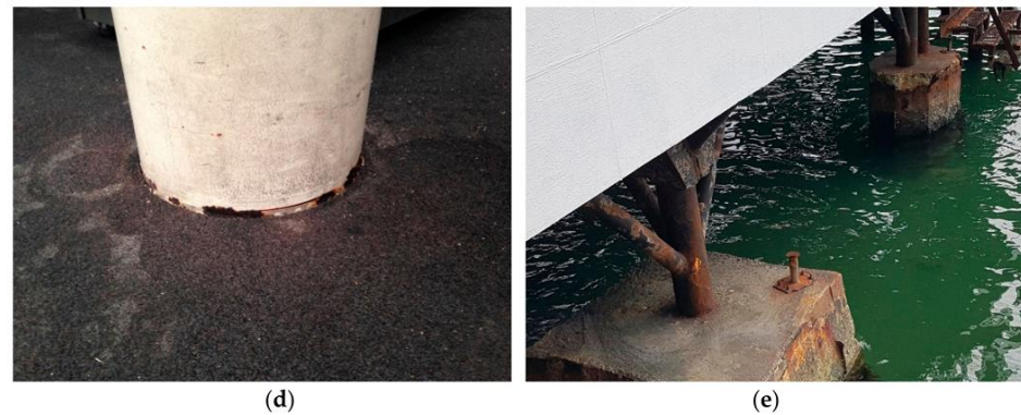
Figure 3. Schematic and field observations of corrosion in short tubular steel columns: (a) different offshore exposure environments; (b) localized corrosion at the ends; (c) corrosion along the column length; (d) observed end corrosion; and (e) observed longitudinal corrosion [57].
