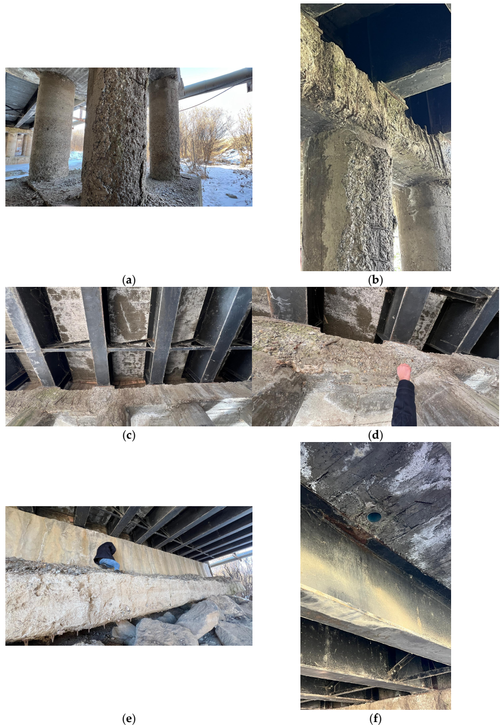
Figure 4. Representative damage observations on the case-study bridge: (a) pier column with cover loss, exposed and corroded reinforcement, and section loss; (b) pier cap beam with advanced spalling and fully exposed reinforcement cage; (c) deck soffit with moisture traces, efflorescence, and calcium deposits; (d) wide cracks and concrete disintegration at a bearing seat; (e) displaced riprap and suspected scour at the western abutment; (f) leakage paths along the deteriorated expansion joint and drainage lines.
