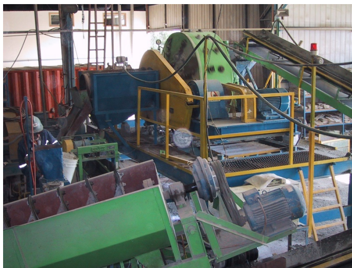
Figure 3. SAG mill, trommel, and spiral classifier.
