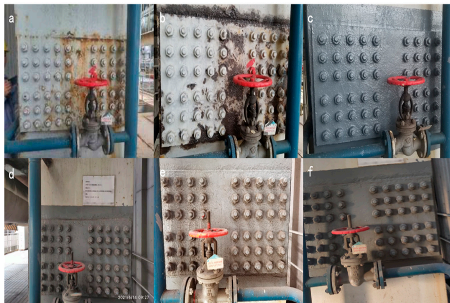
Figure 11. Coatings above boiler connecting bolts: (a) original condition; (b) after rust removal; (c) until 2018; (d) until 2021; (e) until 2022 and (f) until 2023.
