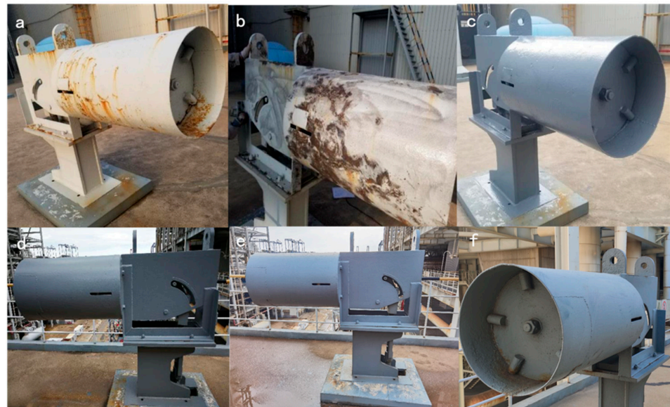
Figure 10. Coatings above spring hangers: (a) original condition; (b) after rust removal; (c) until 2018; (d) until 2021; (e) until 2022 and (f) until 2023.
