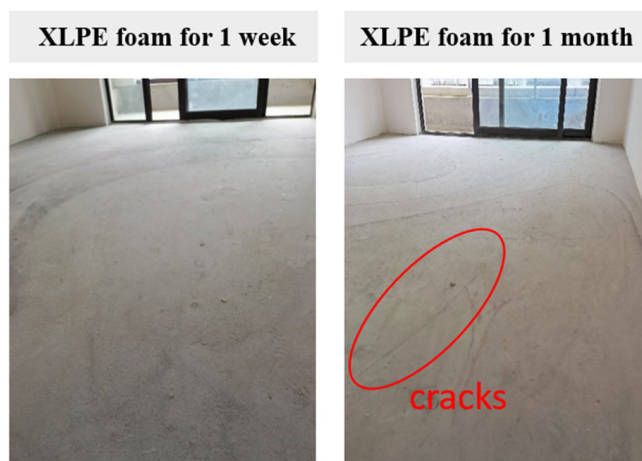
Figure 14. Surface condition of gypsum screeds installed over XLPE foam underlayments under long-term loading.
