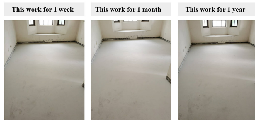
Figure 15. Surface condition of gypsum screeds installed over the composite underlayments under long-term loading.
