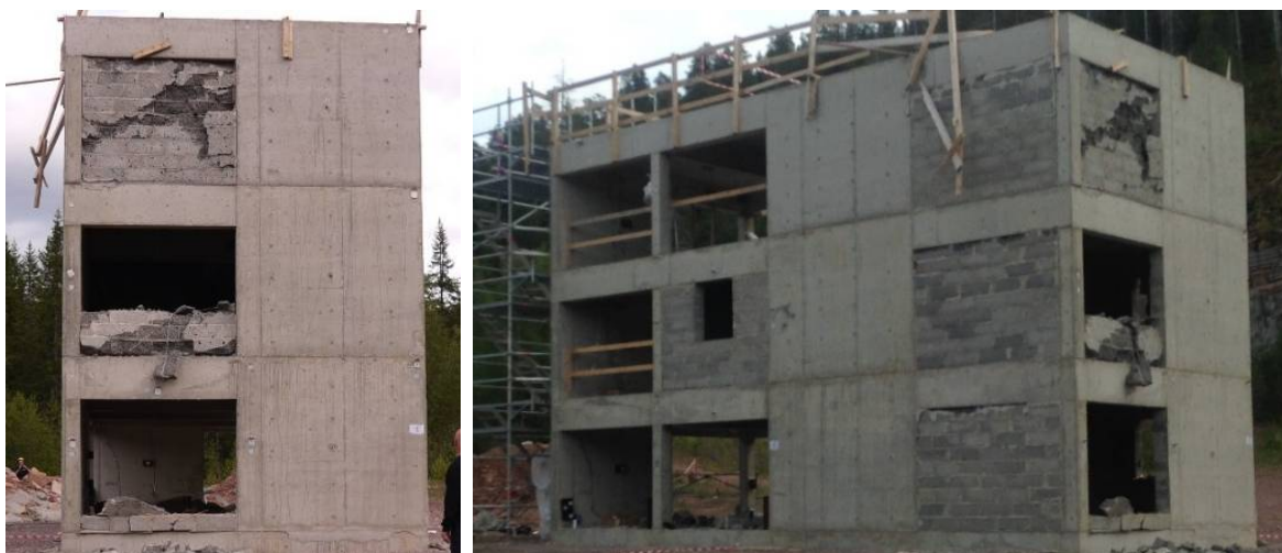
Figure 2. Global damage of the three-story building after the air-blast from front and side view.
