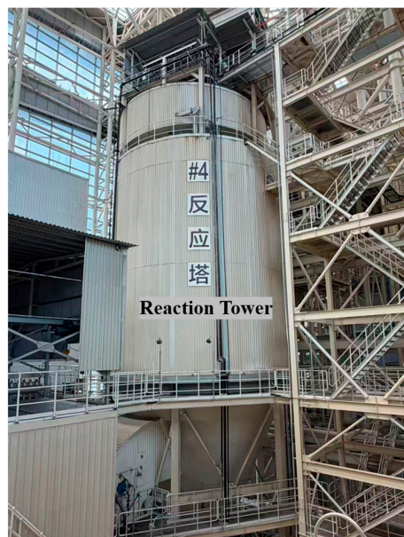
Figure 4. Semi-dry deacidification tower, Shenzhen Energy Environment Co., Ltd.
