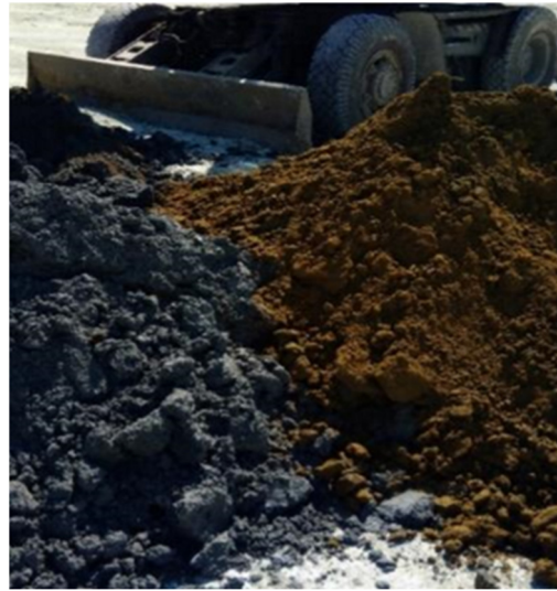
Figure 2. Results of near-surface layer removal on the tailings dump using a wheel loader.
