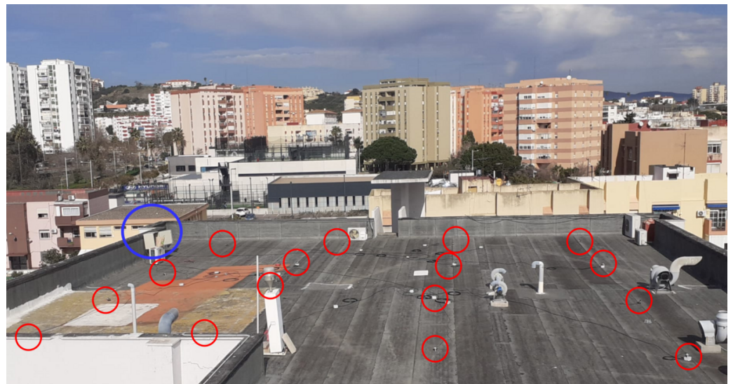
Figure 11. WSN deployed at the rooftop of the University building. Red circles indicate pyranometers, and the blue circle locates the position of the router and AC-DC power supply.
