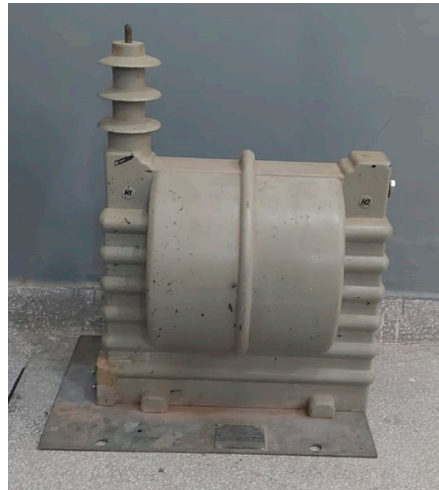
Figure 11. Photograph of the potential transformer.
