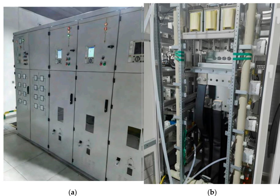
Figure 33. Power cabinet and cooling system of the experimental platform: (a) DC switchgear and DC feeder cabinet, (b) water-cooled heat dissipation bypass thyristor and Crowbar circuit.
