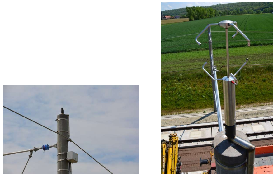
Figure 5. Prestressed catenary pole: (Left) 2D accelerometer; (right) 3D anemometer [25].
