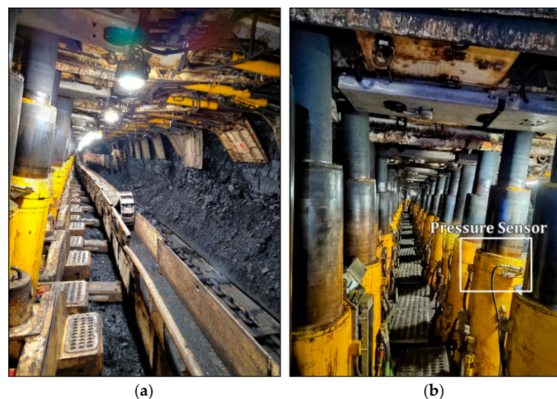
Figure 4. Field monitoring environment and pressure-sensing installation on the hydraulic support. (a) Underground layout of hydraulic supports in the 1503 fully mechanized longwall face. (b) Local hydraulic-oil pipe and connector region where the pressure sensor is installed.
