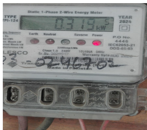
Figure 6. Domestic single-phase electronic energy meter deployed by LESCO for data acquisition.
