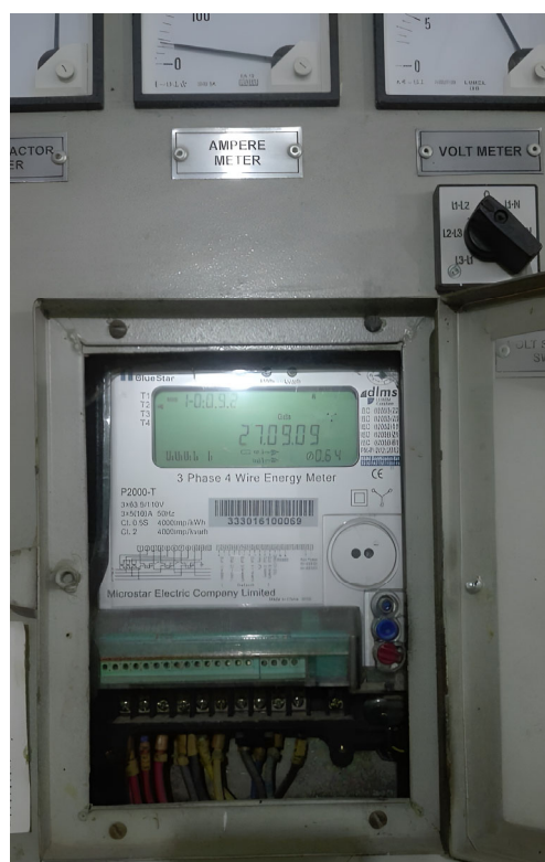
Figure 5. Close-up view of the sensor-based feeder metering infrastructure used for data acquisition in the proposed load forecasting framework.
